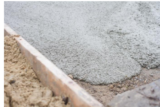
The leading edge of control flow concrete at rest, during placement of a slab-on-ground
